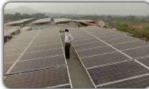
Rooftop Solar Plant
