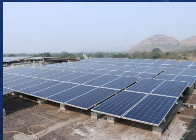
Solar Energy Plant
